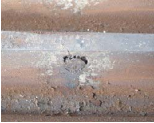
Slag Inclusion Defect
