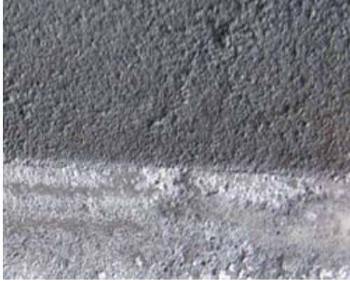
Rough Surface Defect
